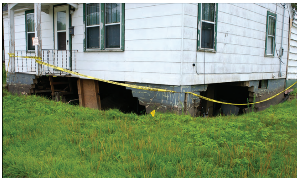
Figure 2-7. The walls of this basement in Wisconsin failed because of the pressure exerted by water and saturated soil.
