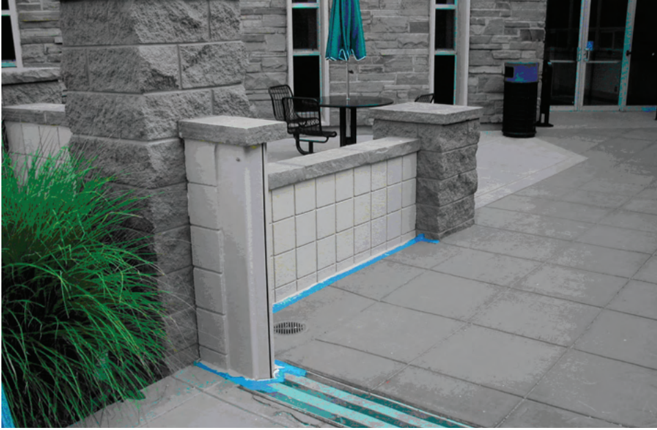
Figure 8-5. The City of Boulder, CO, installed a “pop up” closure to this floodwall at a City office building subject to flash floods. The closure floats up into place automatically when the site is flooded.
