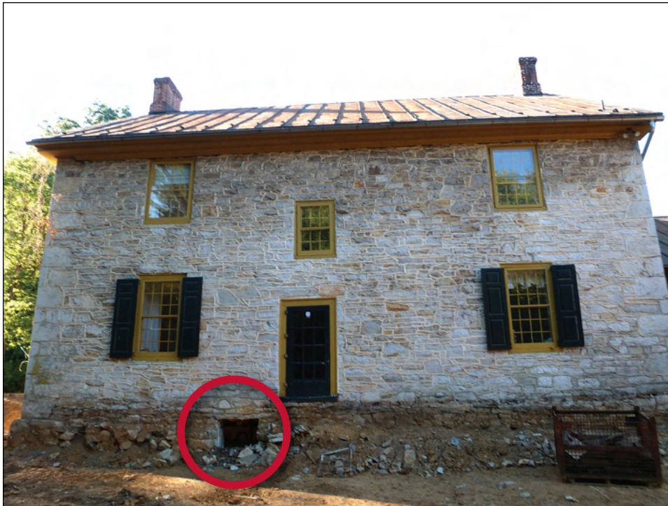
Figure 6-2. Clearing pathways beneath the structure for lifting supports (photo courtesy of Wolfe House Movers).
