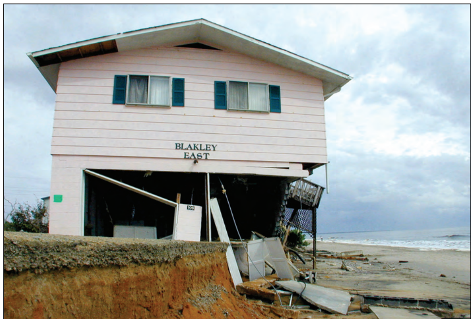
Figure 2-4. The extreme impact of large, fast-moving waves, combined with the removal of supporting soil by erosion and scour, can have devastating effects on buildings exposed to coastal flooding. Hurricane Floyd destroyed this home along the coast of North Carolina in 1999.
