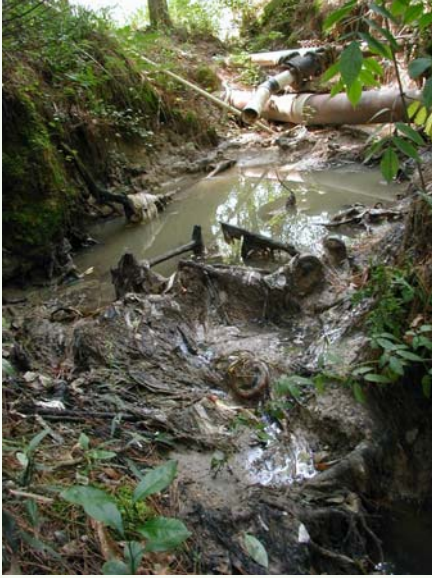
Figure 7-10, Raw Sewage in Ditch
